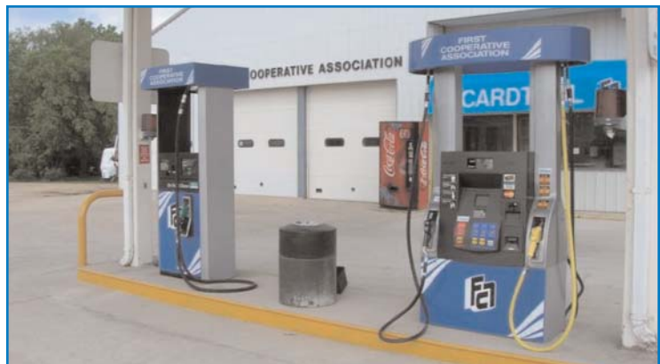
The newly designed fuel pumps installed at the FCA Sioux Rapids location have enhanced the overall appearance of the facilities, and as the top photo shows, now give the customer a choice of 4 grades of ethanol plus B2 bio-diesel.
