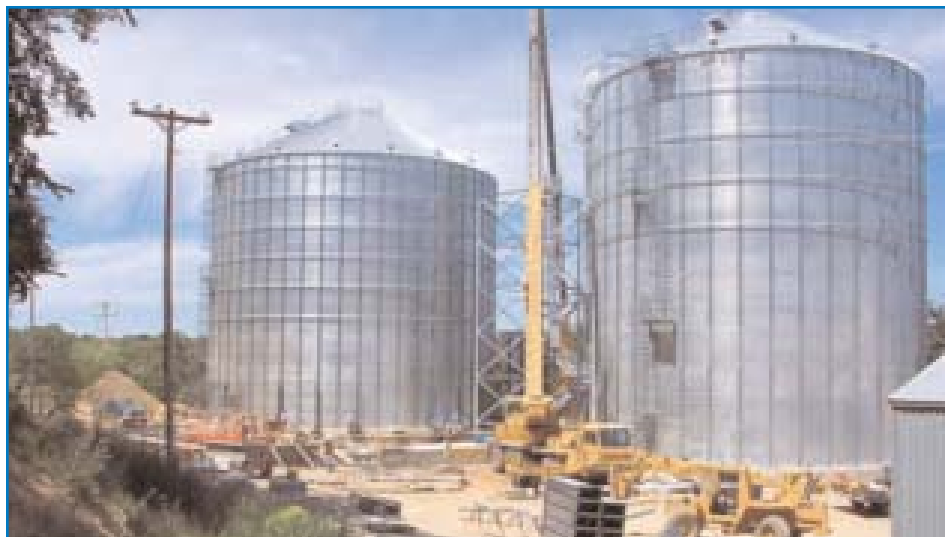
Work is continuing at a rapid pace as we put the finishing touches on the upgrade and expansion projects for of the Linn Grove grain receiving and storage facilities so we can have everything ready to serve FCA customers this fall.
