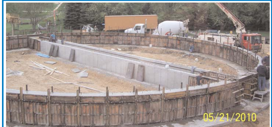
Construction is underway on a new 500,000 bushel steel bin at the Larrabee location of your First Cooperative. The addition of this bin will allow us to designate one of the smaller bins to handle beans in the fall so we'll be able to receive both crops more efficiently.
