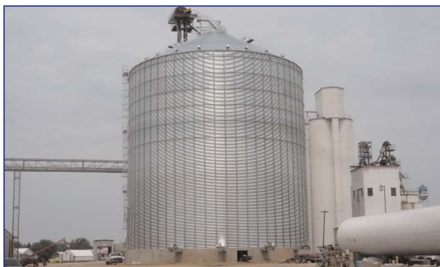
Work on the new 500,000 bushel storage bin at the FCA Aurelia location was just being completed as we went to press in early June. In addition to expanding storage capacities at the FCA Aurelia location with this bin project, we have also installed a new 7,000 bushel per hour grain dryer, which will significantly enhance efficiencies in handling higher moisture corn.
