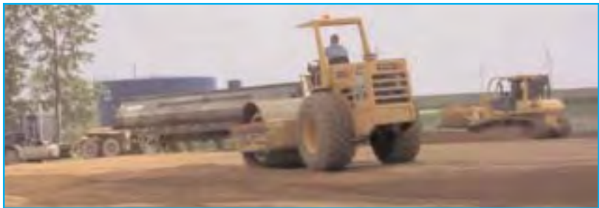
Excavation work was continuing on the new bulk fertilizer plant at the FCA Aurelia location as tons of dirt were being moved and sand was being hauled in to prepare the storage facility foundation.
